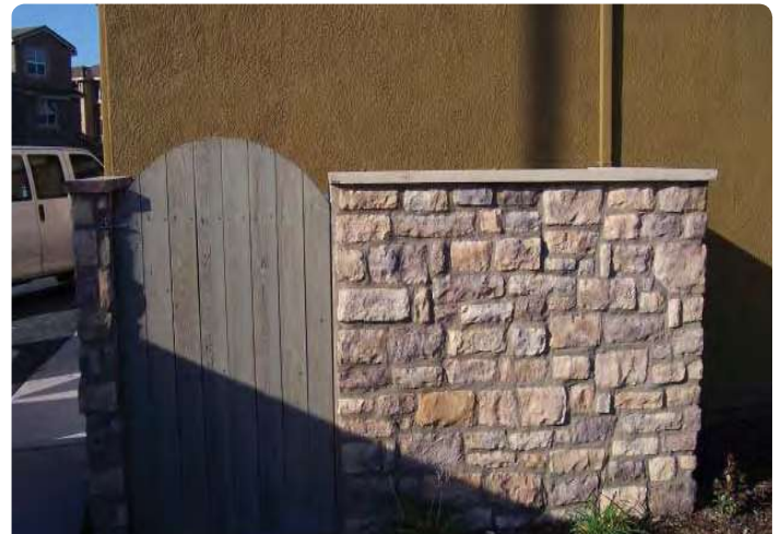
Utility meters effectively screened from view.
